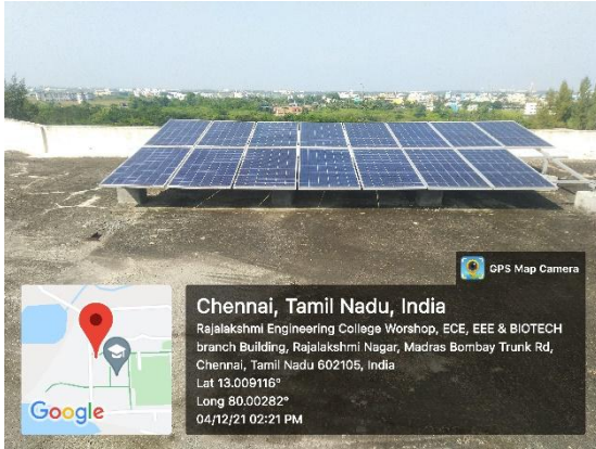
5kW PV panel on rooftop of workshop block
